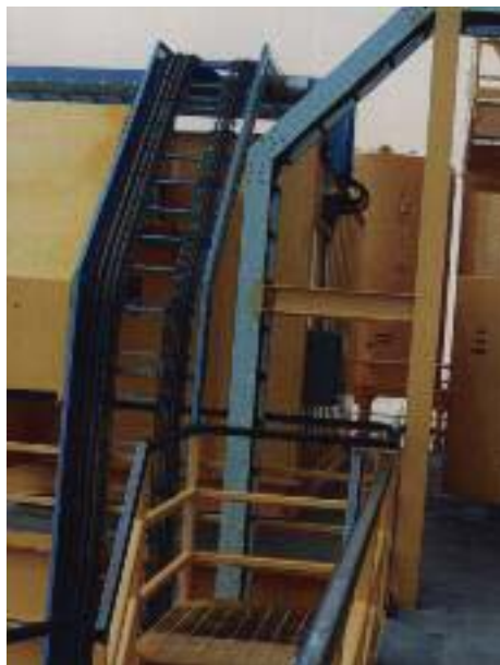
Vertical cable dropout from horizontal run
